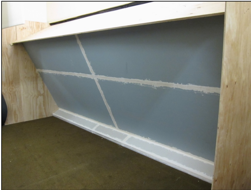
Figure 6: Semi-anechoic side of the roof system construction showing the plywood frame around the ceiling for the sound intensity measurements. The ceiling was made of plasterboard and the seams were sealed with paper and plaster.
