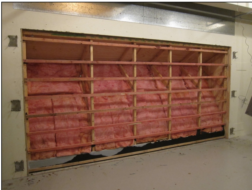
Figure 7: View from the reverberation room of the sound absorbing materials installed above the ceiling.
