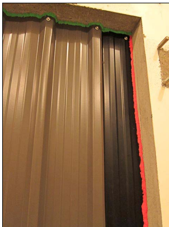
Figure 8: Sealing compound around the edges of the cladding to prevent sound leakage around the edges of the cladding.
