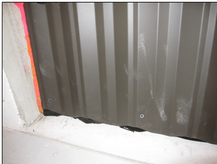
Figure 9: Resilient material located between the bottom row of tiles and the concrete floor.
